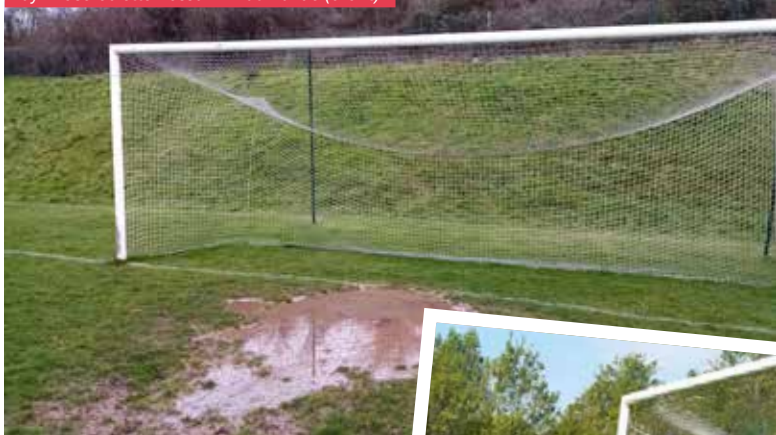
Gymnase Colette Besson - But inondé (avant)
